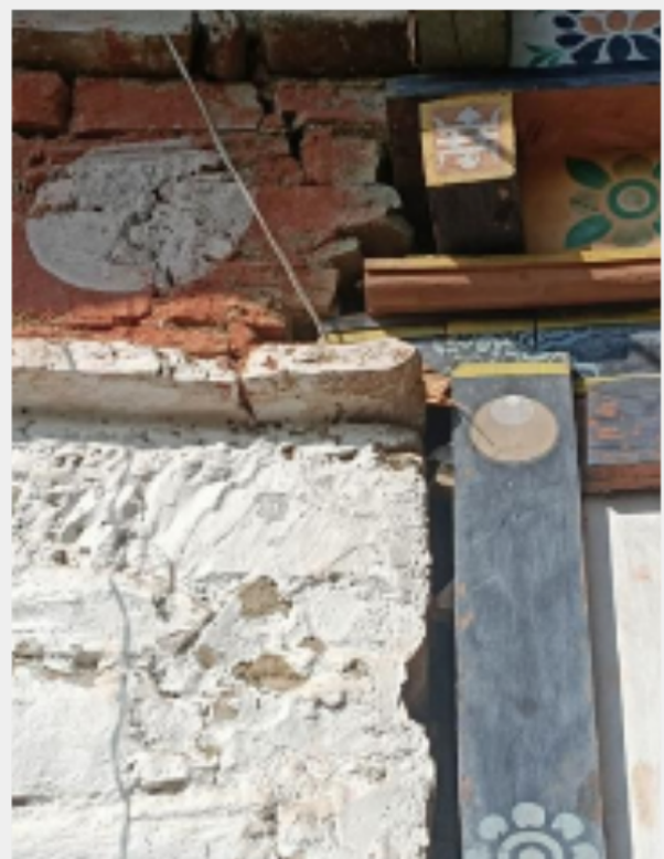
Minor cracks caused by the earthquake.
