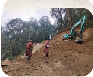
Construction of Wama- Khomsar road connecting Mongar and Zhemgang DZongkhags to boost ecotourism.
